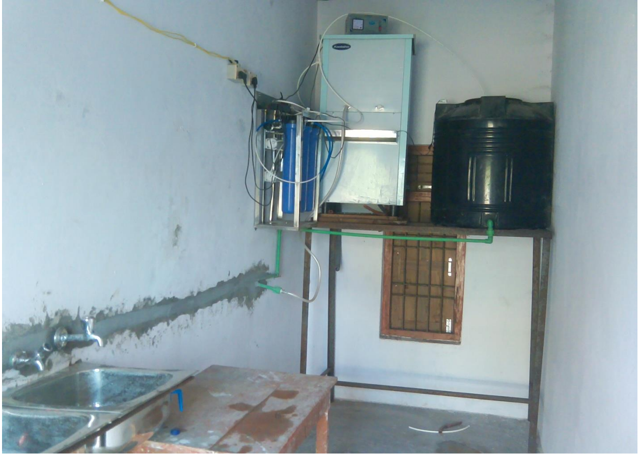
Annex-38 (Relating to Question No 80 of Criteria 5) Photo of water purifying machine, water tap & Toilet
