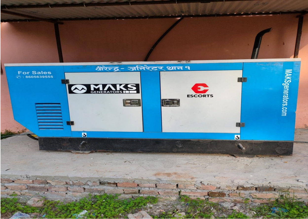
Photo of Generator
