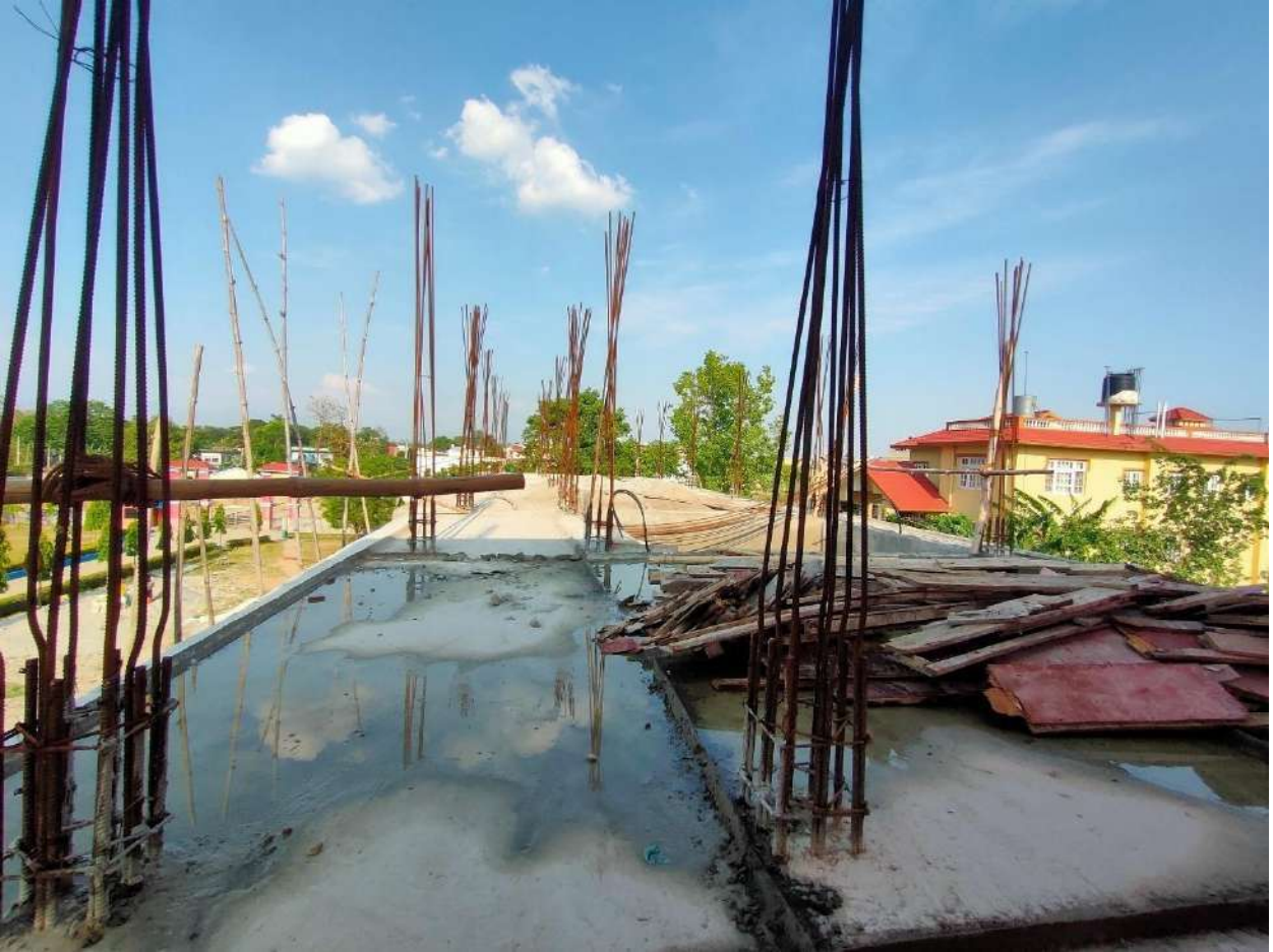
Annex-114 (Relating to Recommendation No 1 of Criteria 5) Photo of e-library building under construction.
