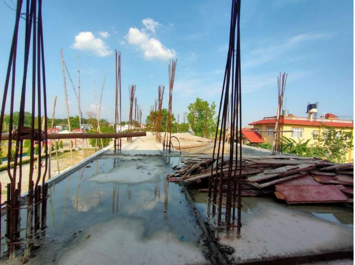
Annex-105 (Relating to Recommendation No 5 & 7 of Criteria 5) Photo of e-library building under construction
