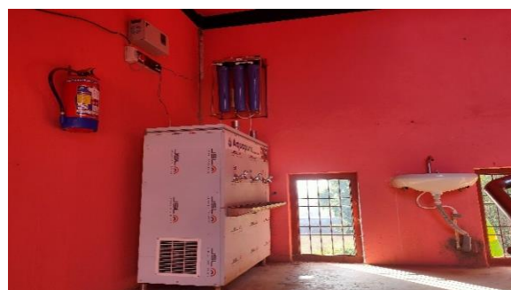
Water Purifier & Refrigerator for Drinking Water
